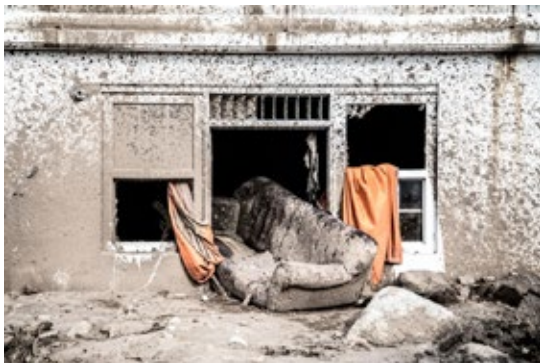
Photo credit: Tomás Ayuso/Irin. Impact of Hurricane Maria flood waters on a house in Dominica, September 2017.
